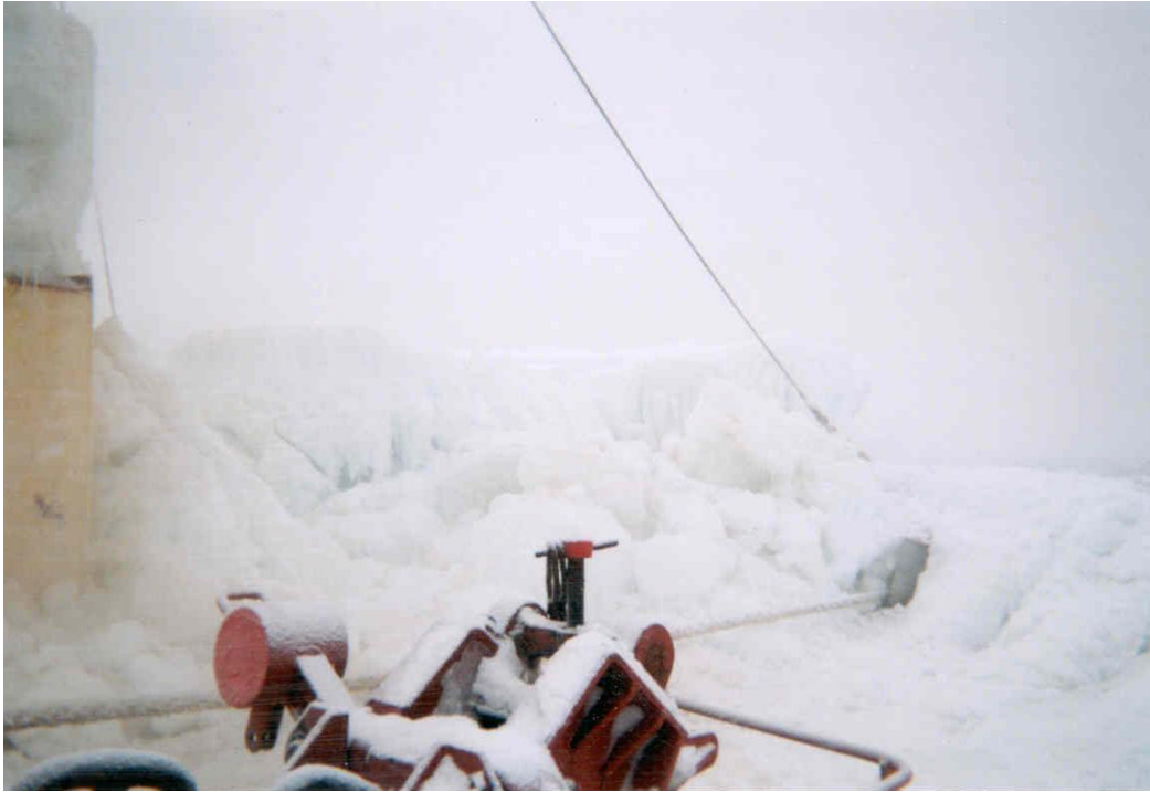
Figures 5.3I– Guy wire view after de-icing
